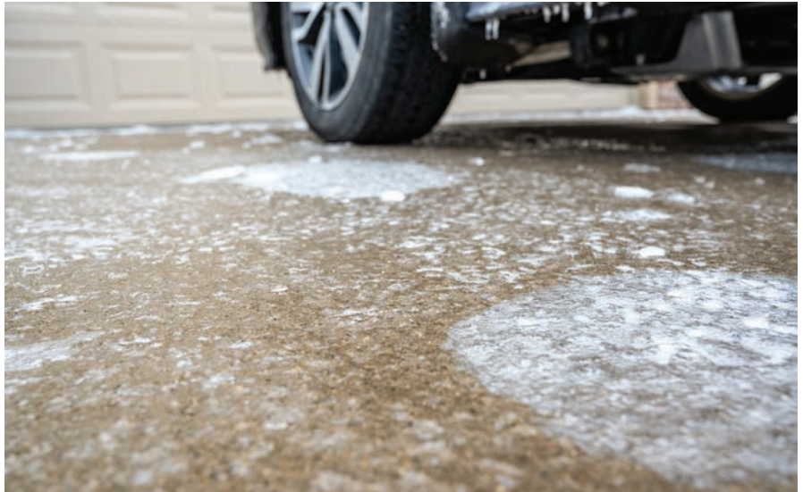
Sensors in snow melt systems can detect snow or ice on the pavement and trigger the process.
